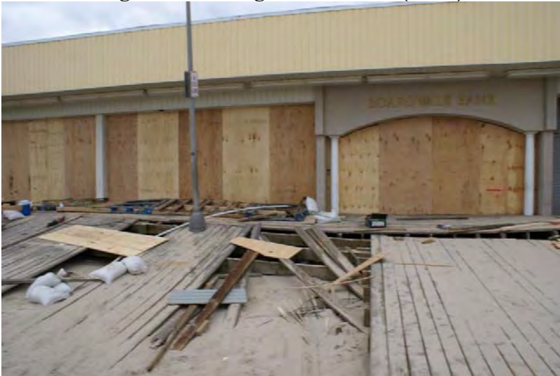
Figure 10: Damaged Boardwalk (2 of 2)
