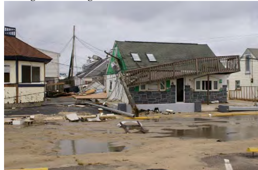
Figure 4: Damaged House and Downed Power Line
