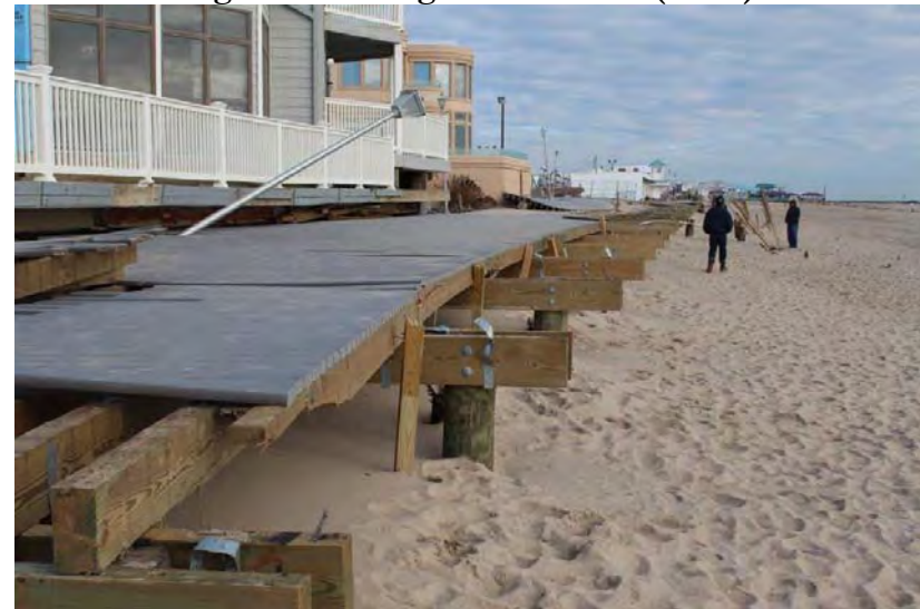
Figure 9: Damaged Boardwalk (1 of 2)
